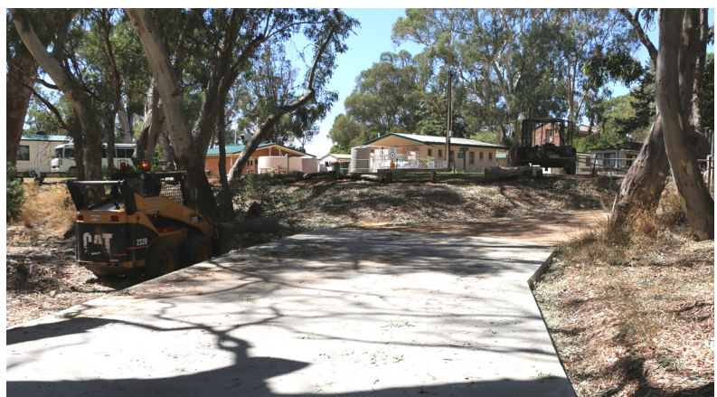
Joies Road creek crossing in Melrose has been replaced. Council allocated funds towards this project in the 2017/2018 Annual Budget.
