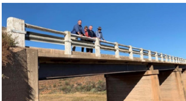
Mount Remarkable Mayor Phillip Heaslip, Cr Denise Higgins and Mayor Ben Browne (Northern Areas Council) with Member for Grey Rowan Ramsey MP at the Pine Creek Bridge.
