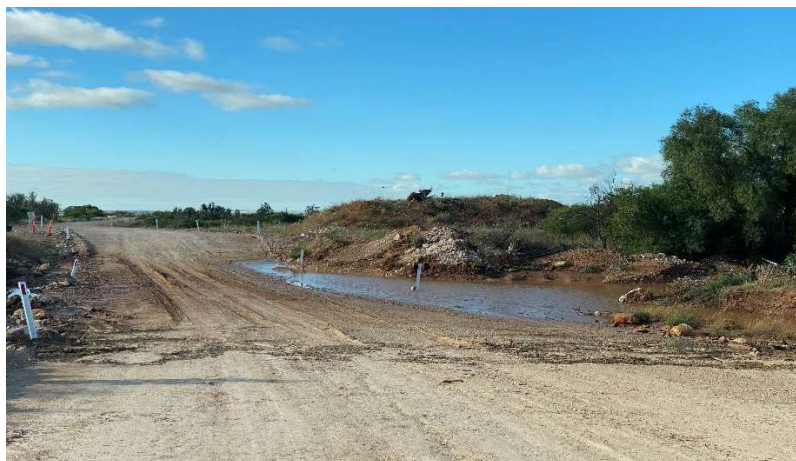
Willowie Creek Flooding
